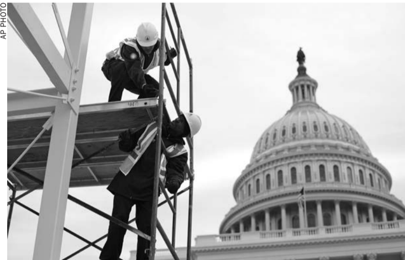
In this Dec. 8, 2016, file photo, construction continues for the Inauguration and swearing-in ceremonies for President-elect Donald Trump on the Capitol
